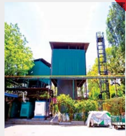
Biogas system, MIL Hapur
