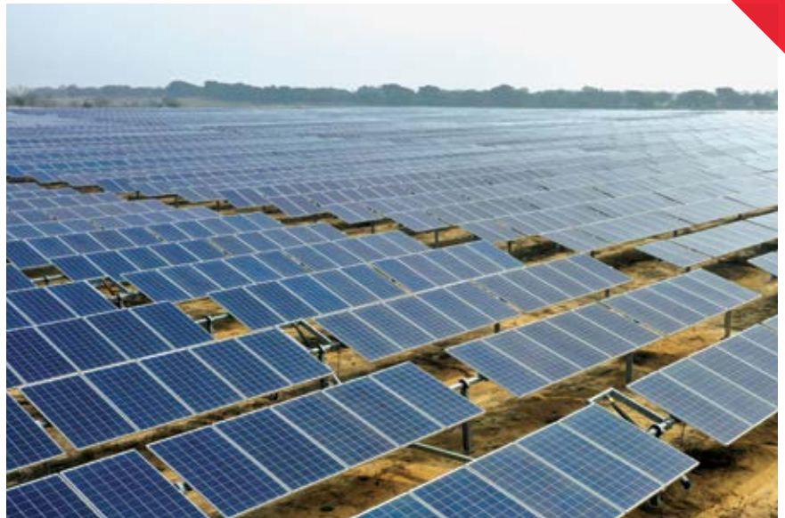
Groundmounted Solar System - Merino Rohad (H.R.)
