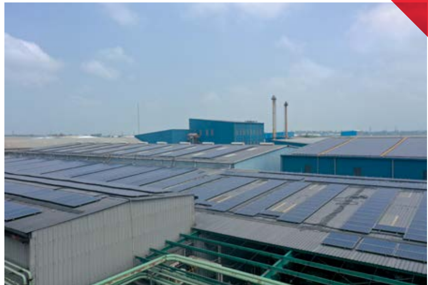
Rooftop Solar System MIL Rohad (H.R.)
