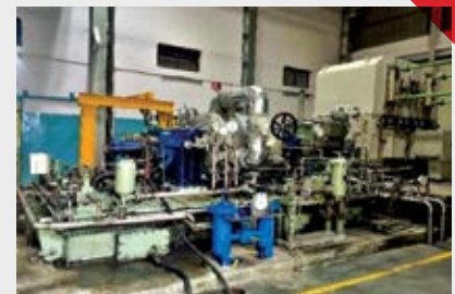
Biomass based Turbine, Hapur
