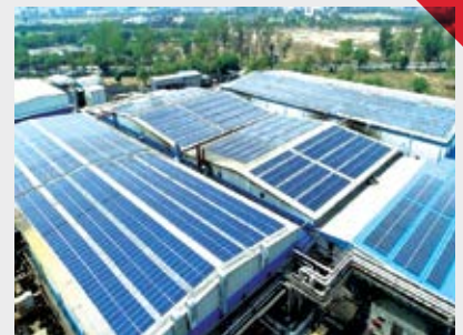
Rooftop Solar, MIL Hapur
