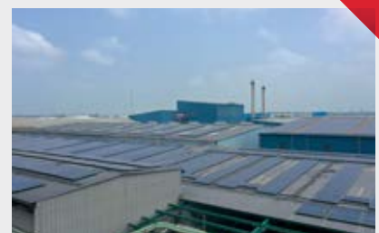
Rooftop Solar, MIL Rohad
